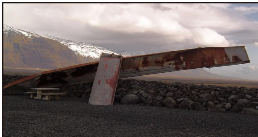
Figure 8.1: Photograph of remains of bridge damaged by the jökulhlaup associated with the 1996 Gjalp eruption under Vatnajökull, see picnic bench for scale.
