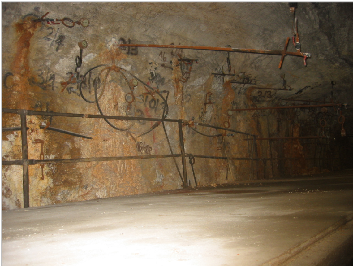
Figure 3-4: Boreholes at the internal seepage site LS1 H23 on the 470 m level (Photo U. Argut).
