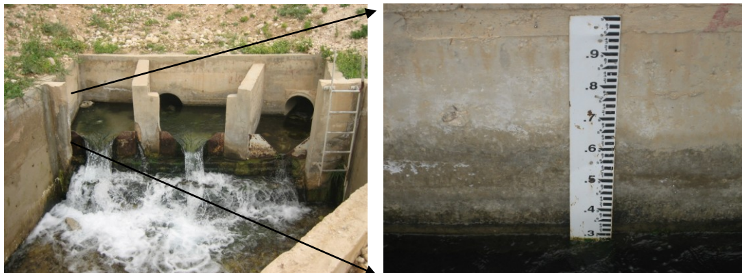
Fig. 5.9: Seepage from Kafrein dam reservoir measured using a V-notch and a stage height (Photo taken on 16 th of April, 2007).
