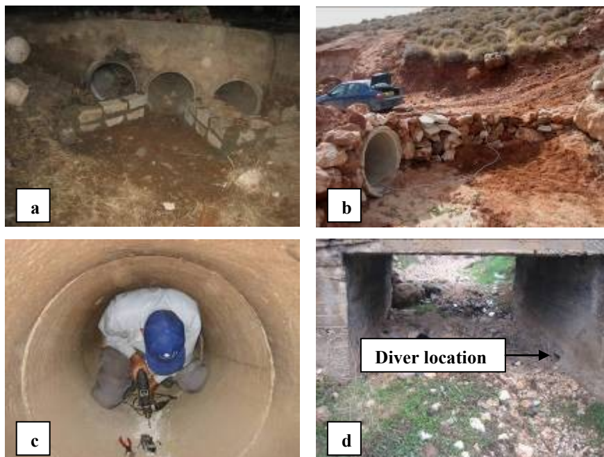
Fig. 4.19: a. Construction work in Wadi An Nar S4 b. Water diversion to the circular culvert in Wadi Kurnub S5 c. The automatic pressure transducers (divers) were installed inside a metal box and fixed in the bottom of the circular culvert d. Diver installation in Wadi Kuraysh S1
