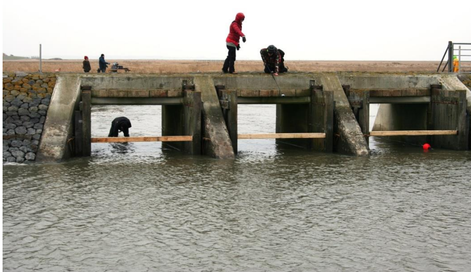
Figure 5-3: Open gates at the tidal channel system “Osterwehl” (Langeness). Gates are fixed by wooden beams against a closing by water inflow. Photo by M. Deicke (2013).
