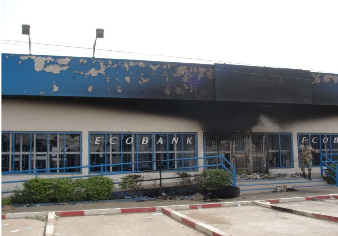
Figure 10: Burned-down ECOBANK at the Total roundabout in Zinder. Taken on the afternoon of December 8, after the military had been deployed to secure the city. Photo: Jannik Schritt
