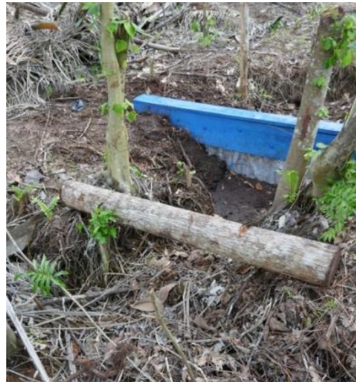
Fig. 8: Dried peat showing a failed attempt to stop drainage with a canal block.
