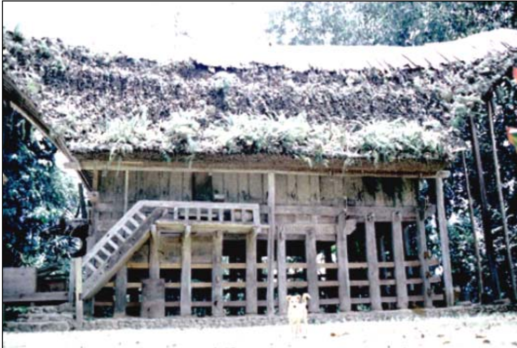
Figure 5.12. Ageing Process decrease the value of old Tongkonan in Tana Toraja (Credit: Avenzora, R)
