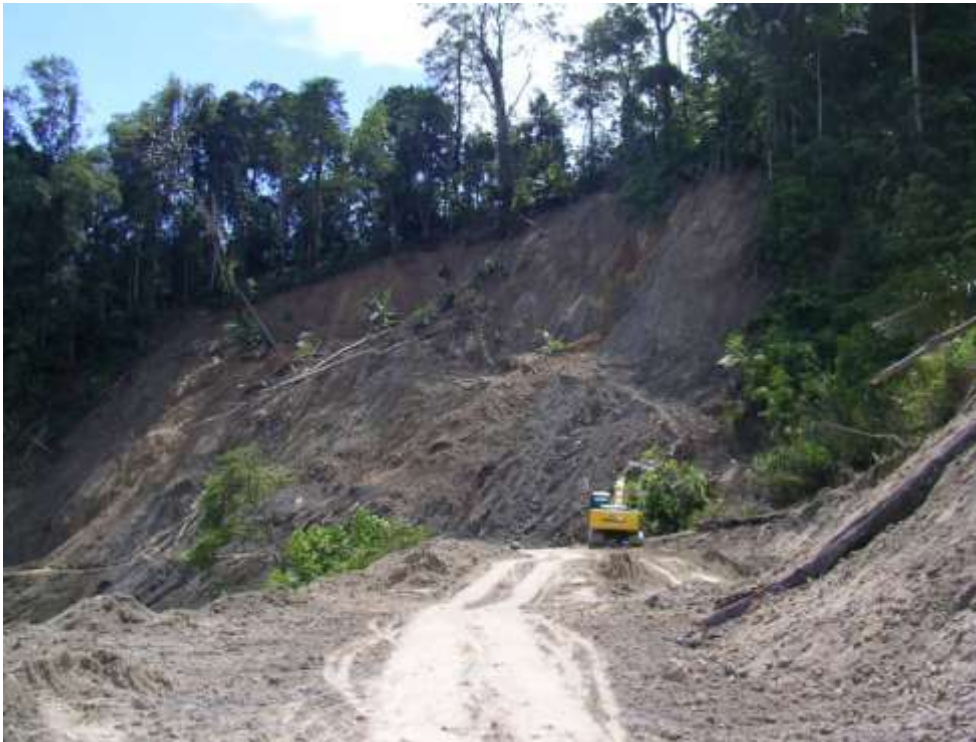
Figure 2.15: Landslide in the Kulawi Valley on the main road to Toro and Lempelero.
