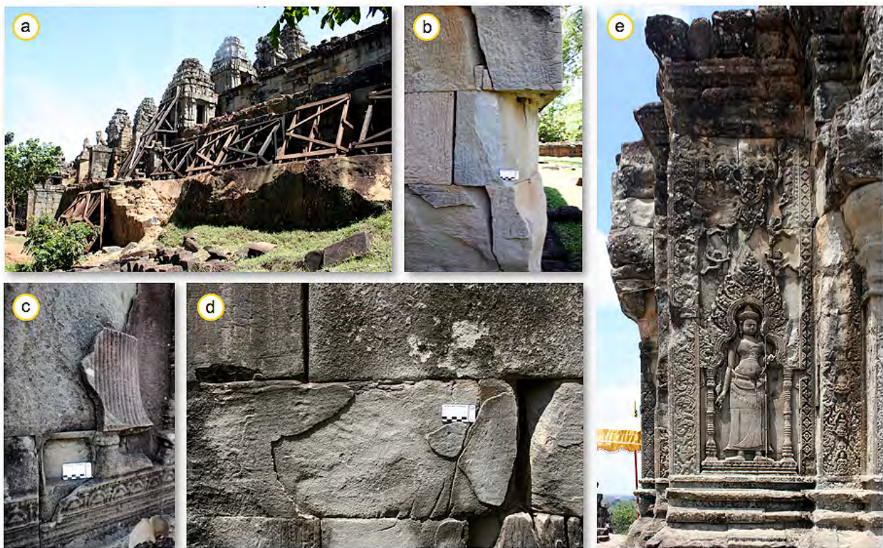
Figure 117: Damages at the Phnom Bakheng Temple: a) wooden protection constructions at the pyramid walls, b) structural cracks, c and d) contour scaling and e) back-weathering at the upper relief zone.
