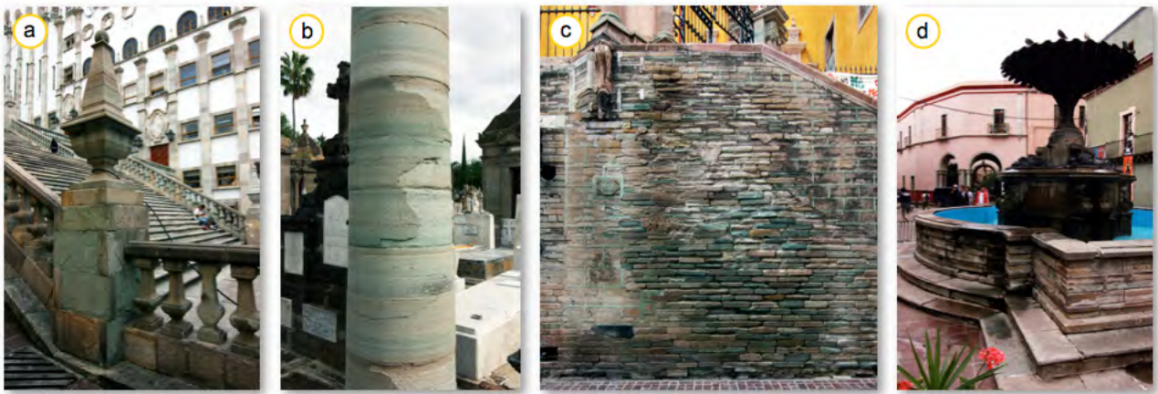
Figure 59: Appearance of the different damage and deterioration types observed in the Loseros Tuff. a) Delamination at the stairway of the main building of the university. b) Contour scaling perpendicular to the lamination at a column of a tomb in Guadalajara. c) Flaking and crumbling in the lower part of a wall affected by moisture infiltration and d) at a basin wall of a fountain in Guanajuato.
