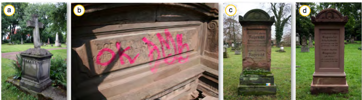
Figure 185: Vandalism and destruction at several tomb monuments at the Bartholomew Cemetery. a) Mechanical violence, b) graffiti and c) the historical Rubrecht Tomb and d) the reconstructed one.
