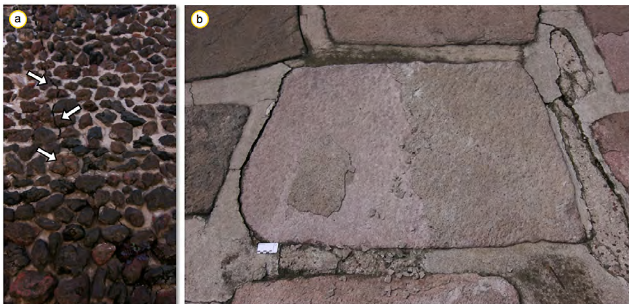
Figure 45: a) Structural cracks observable in the tezontle (arrows) and b) scaling of tenayocátetl plates parallel to the surface.
