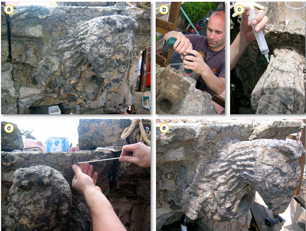
Figure 182: a) A gargoyle before conservation. b) Drillings for the fiberglass sticks. c) Cleaning and consolidation of the flanks of the cracks. d) Application of the fiberglass sticks and e) the gargoyle after consolidation and conservation.
