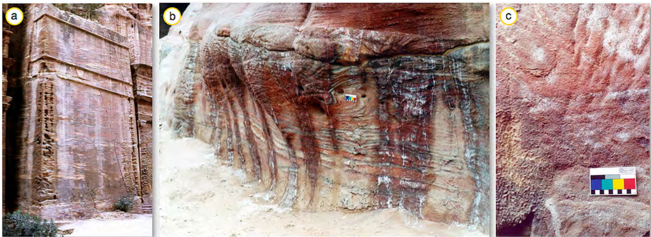
109: a) Wet area due to hygroscopic salts at one monument along the streets of the facades, b) water drainage and salt efflorescences and c) salt efflorescences at monument no. 826 after a heavy rainfall.
