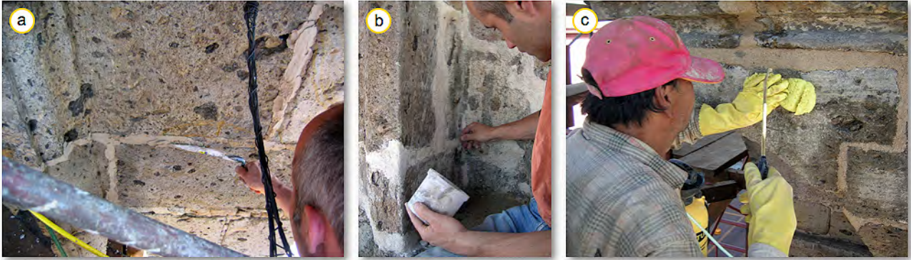
Figure 184: a) Application of the jointing mortar, b) egalization after hardening and c) after-treatment of the surface by wetting and washing.
