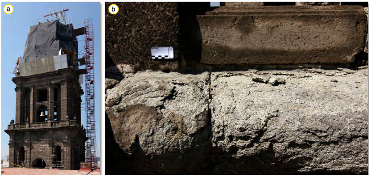
Figure 49: a) The left tower of the cathedral under restoration in 2009. b) Typical weathering forms consisting of gypsum crust formation, scaling and rounding of a sculpture at the Metropolitan Cathedral.
