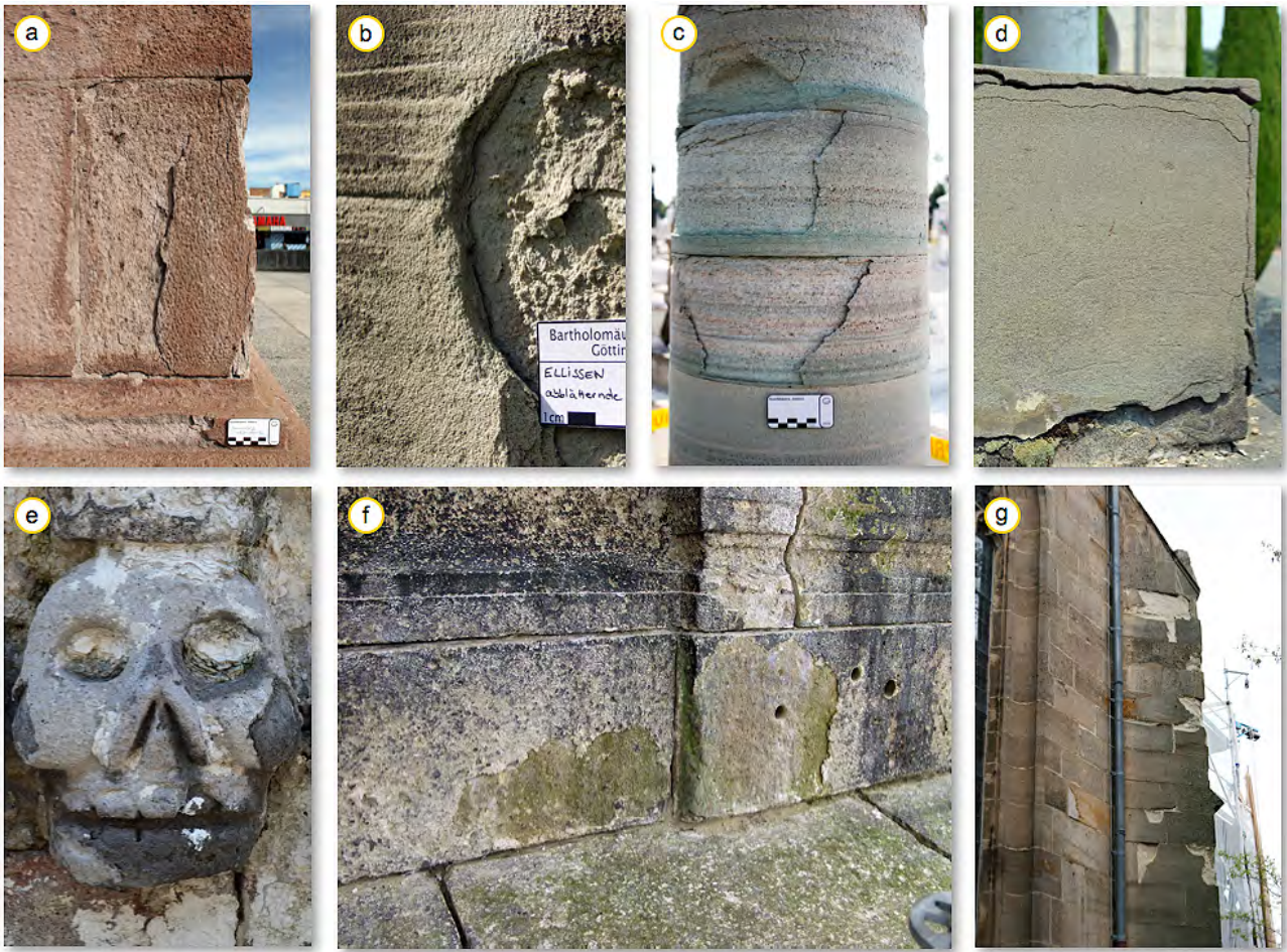
Figure 19: a) Scale formation due to gypsum accumulation at the monument of independence in Guadalajara, Mexico (tuff), and b) perpendicular to the bedding due to gypsum accumulation at a sandstone tomb in Göttingen, Germany. c) Contour scaling perpendicular to the bedding due to calcite accumulation at a tomb in Guadalajara, Mexico (tuff). d) Massive crust formation and contour scaling at a tomb in Lugano, Switzerland (clay-rich sandstone). e) Contour scaling due to hydrophobization at the Templo Mayor in Mexico City, Mexico (tuff), and f) at the Charlottenburg Gate in Berlin, Germany (tuff) as well as g) at the Servatius Church in Duderstadt, Germany (sandstone).
