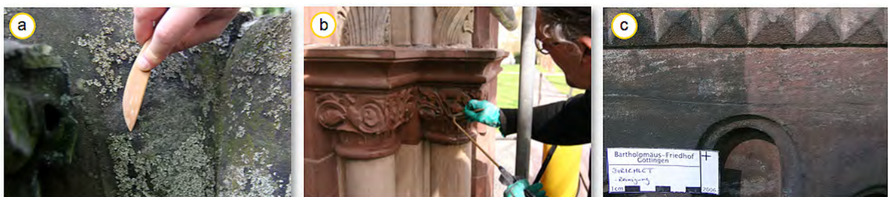
Figure 33: a) Cleaning of microbiological growth with a wooden tool. b) Wet cleaning of dust and loose deposits. c) Cleaning effect by using the micro-abrasive method on sandstone.
