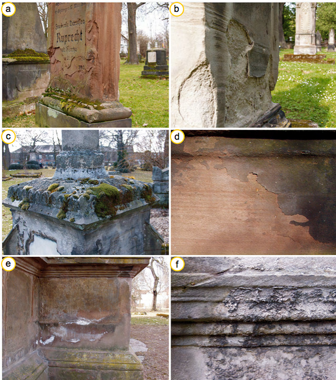
Figure 93: Typical weathering forms of the sandstones from the Bartholomew cemetery in Goettingen: a) scaling parallel to the bedding; b) contour scaling perpendicular to the bedding with secondary detachment of small flakes; c) biological colonization; d) flaking combined with black crusts; e) salt efflorescences; and f) formation of gypsum crusts.
