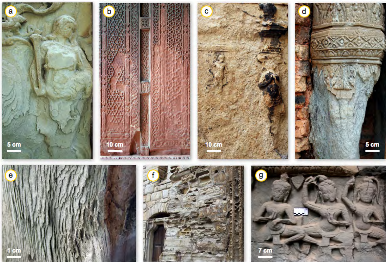
Figure 16: Weathering phenomena in sandstones: a) delamination parallel to the surface (Zeitz, Germany). b) Sanding parallel to the surface (Fatehpur Sikri, India). c) Flaking (Wittenberg, Germany). d) Crust formation, cracking and lamination parallel to the bedding (Angkor, Cambodia). e) Lamination parallel to the bedding (Goettingen, Germany). f) Alveolar weathering (Zeitz, Germany). g) Cracking and contour scaling (Angkor, Cambodia).
