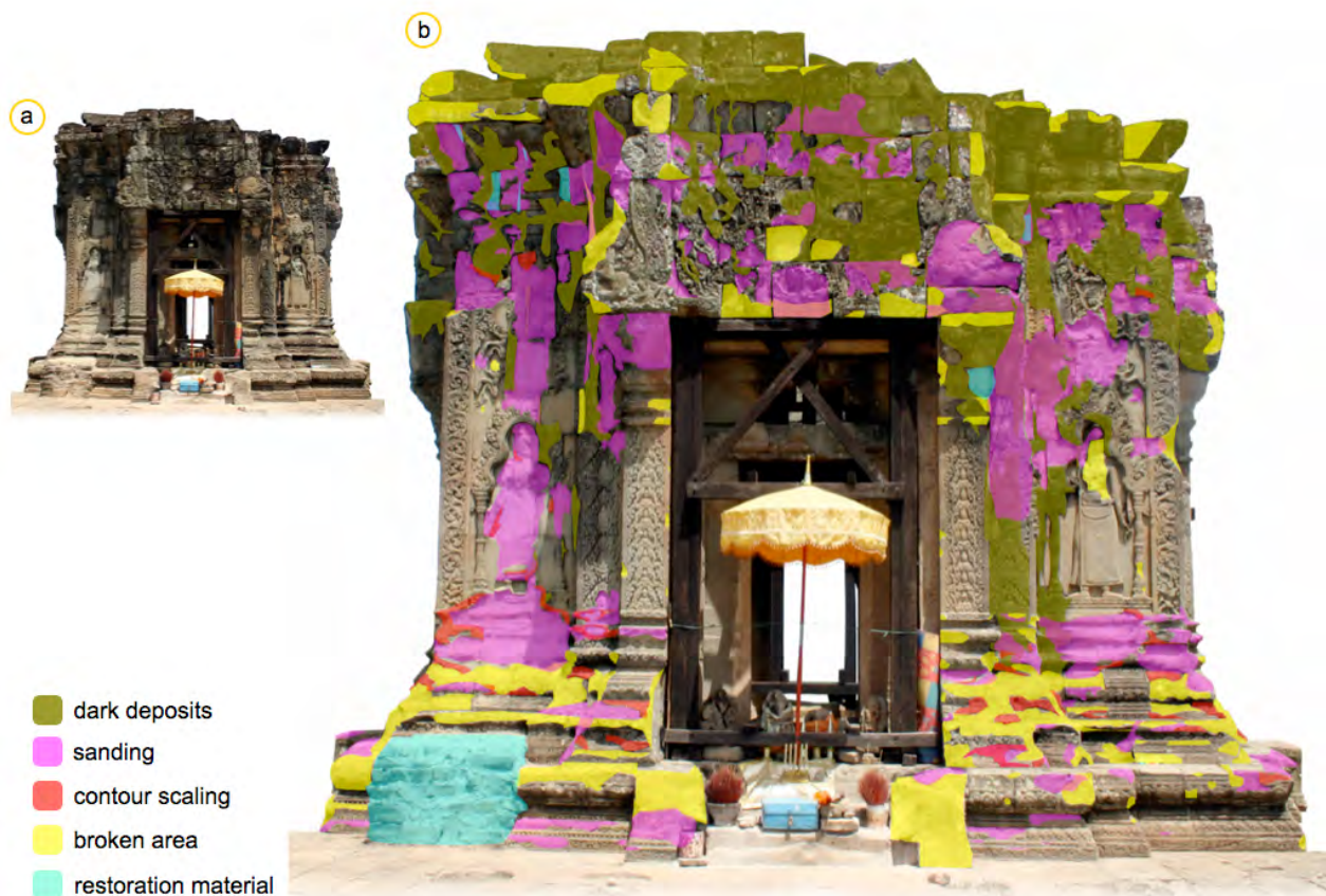
Figure 121: Quantified mapping of the south facade of the main sanctuarium of the Phnom Bakheng Temple. a) The conservation state of the facade and b) quantified mapping.
