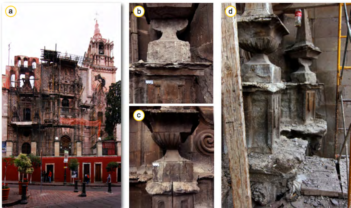
Figure 60: Massive deterioration of the Bufa Tuff at the Compañía de Jesús Church. a) The church under construction, b and c) structural cracks in detail at a pillar in the facade and d) the weathering situation at the facade.
