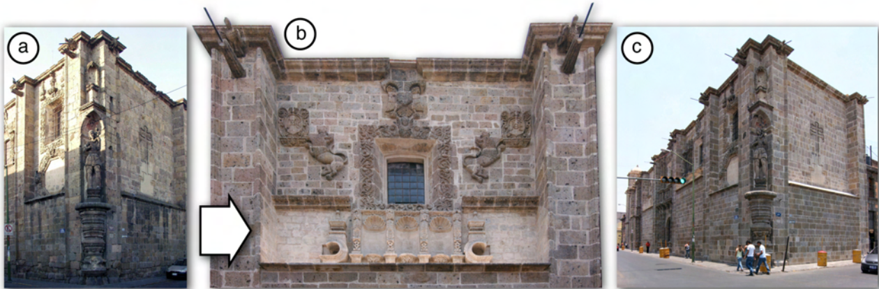
Figure 75: a) Church before restoration. b) Area where architectural elements were discovered (arrow) that include three niches for the placement of religious sculptures. c) Church after restoration.
