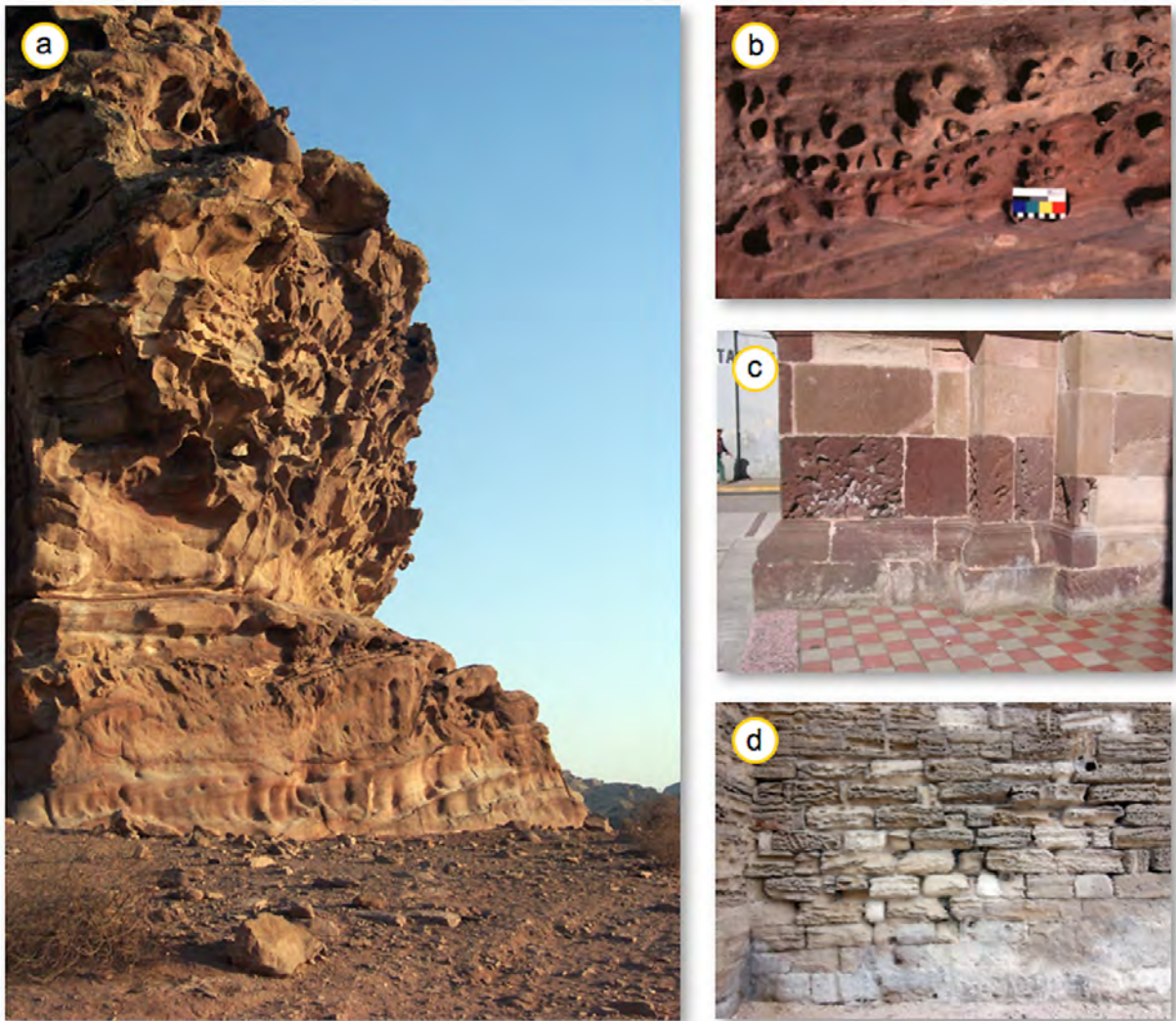
Figure 18: Tafoni and alveolar weathering. a) Tafoni weathering in the region of Petra (Jordan), b) alveolar weathering in Petra, c) alveolar weathering of tuff at the San Francisco Church in Zamora, Michoacan/Mexico and d) alveolar weathering at the historical city wall of Avignon (France).
