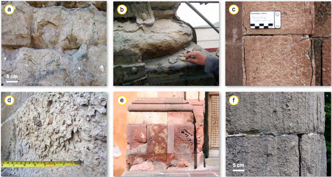
Figure 17: Weathering phenomena in tuffstones. a) Structural cracking and scaling (Rome, Italy). b) Cracking and scaling parallel to the surface (Berlin, Germany). c) Cracking and crust formation (Guadalajara, Mexico). d) Structural flaking (Guadalajara, Mexico). e) Alveolar weathering (Guanajuato, Mexico). f) Disintegration parallel to the surface (Kassel, Germany).
