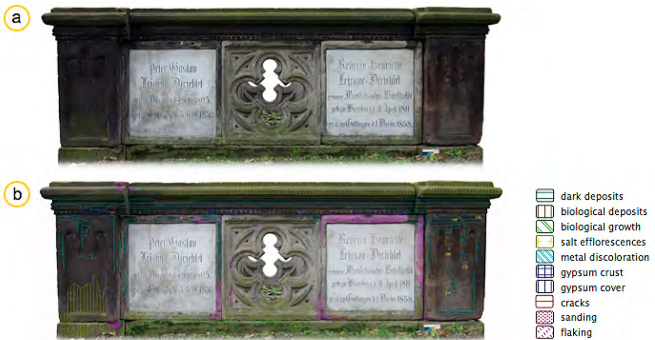
Figure 97: a) The Lejeune-Dirichlet Tomb before conservation/restoration and b) damage mapping.
